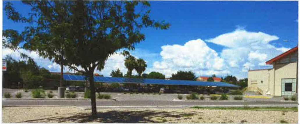
Ameresco installed 181.2 kW-DC amongst two solar photovoltaic carport canopy arrays covering 60 parking stalls.
